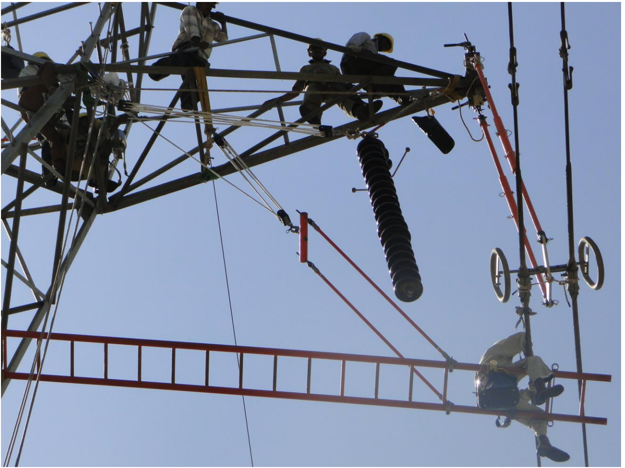
400 KV Suspension Operation
