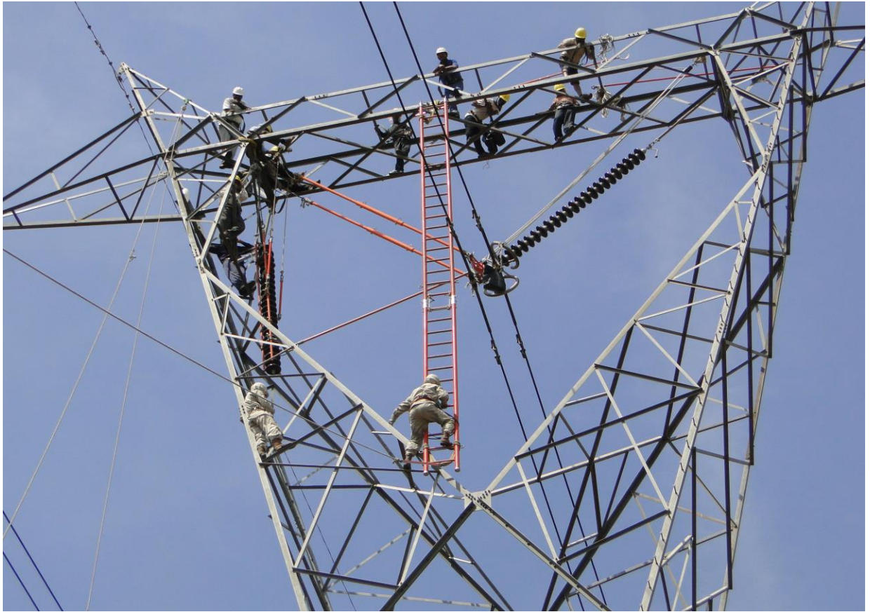
400 KV "V" String Operation
