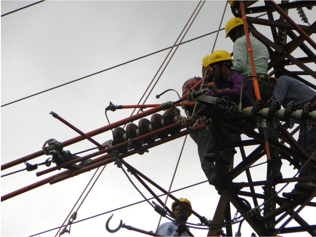
66KV Tension Operation
