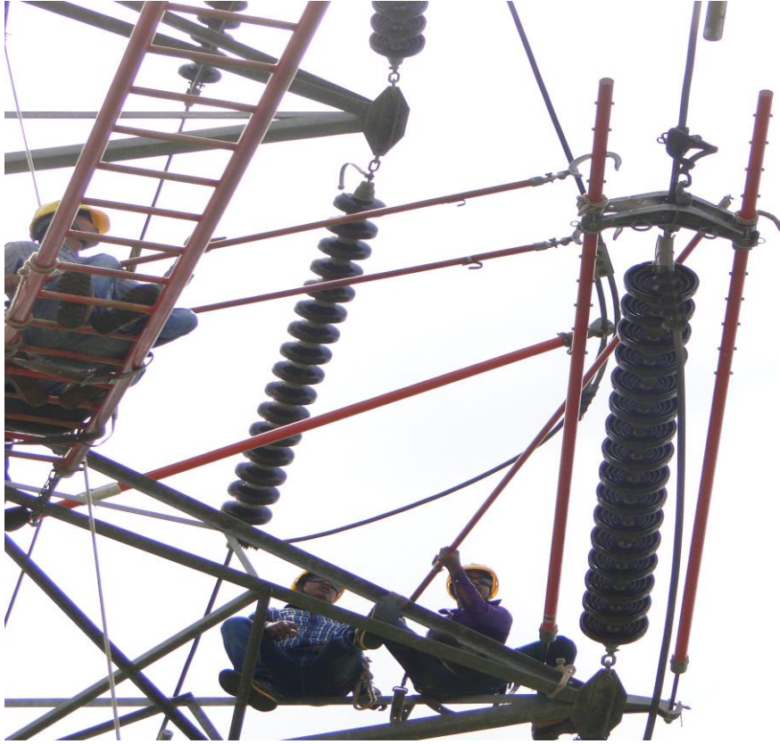
220 KV Tension Operation
